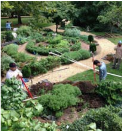
An entirely new irrigation system was installed on the property to better care for our 1.2 acres of landscaped gardens with a total of 40 separate irrigation zones. Advisory Committee member and award winning landscape designer Guy Williams & DCA Landscape Architects advised on the system upgrade
