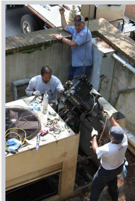
A little less than a year after a direct lightning strike to the chiller caused compressor failure in our HVAC system, an electrical surge after another storm fried the compressor for a second time in the summer of 2014. Upgrading the HVAC system is a top priority in the 2014-2019 Strategic Plan.
